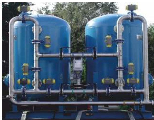
Industrial Water Treatment Plant for Power Industry
