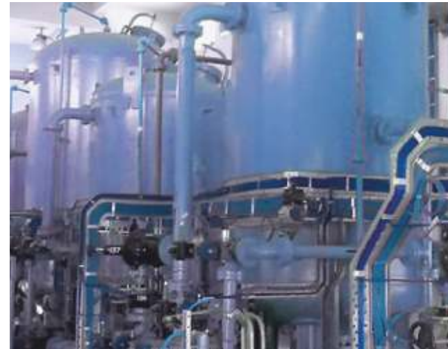
Industrial Waste Water Treatment for Heavy Engineering
