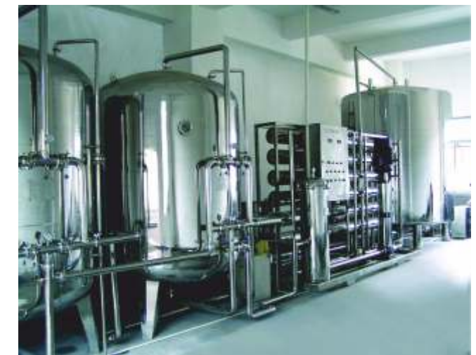
Industrial Waste Water Treatment & Recycling Plant for Engineering
