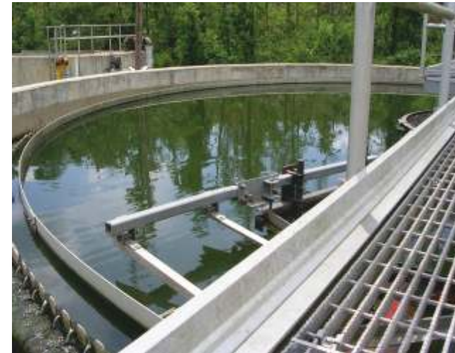
Effluent Treatment Plant for Electronics
