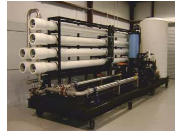
Reverse Osmosis Plant for Automotive OEM
