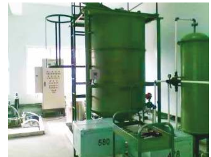
Effluent Treatment Plant for Power Equipment Mfg.
