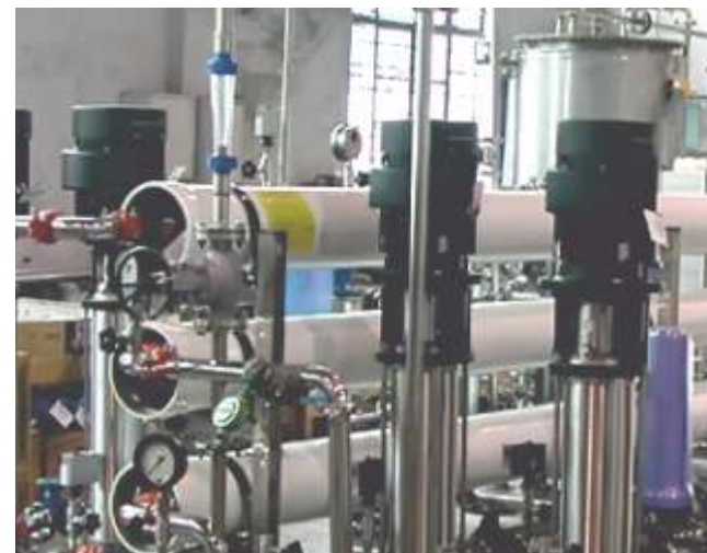
Industrial Waste Water Treatment Plant for Defense
